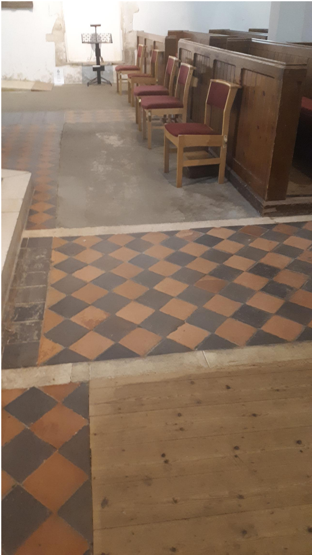
Floor at the front of the nave showing the mix of pine, Victorian tiles and concrete
